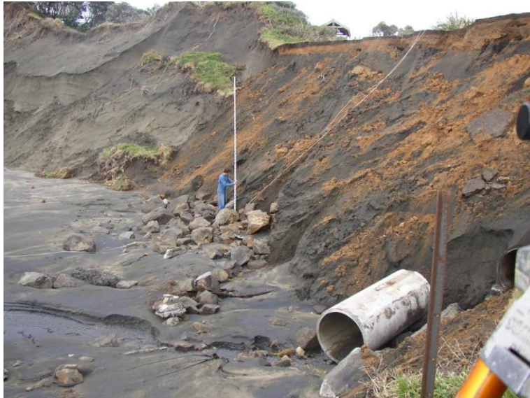
Early erosion of bank, storm water pipe undercut and dislodged from bank. June 2006
